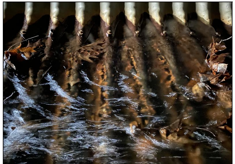
Perforations along Invert below Roadway
