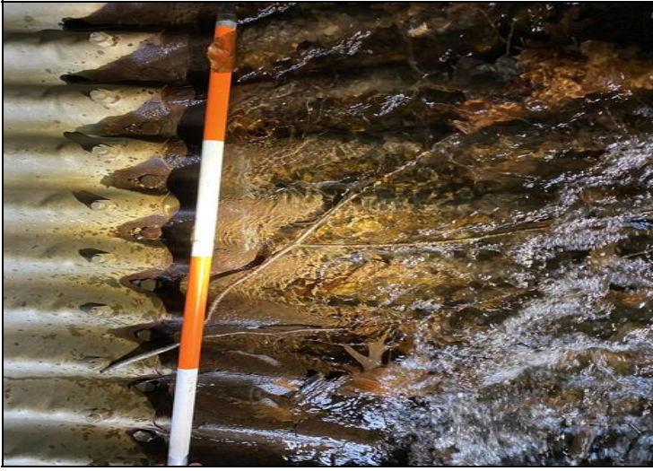
Large Perforations along Southern Side of Culvert Invert
