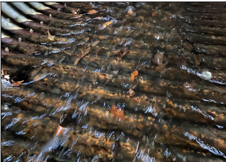
Perforations along Invert below Roadway
